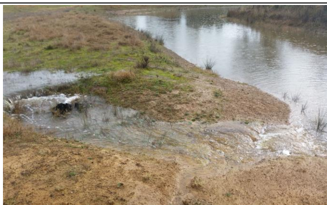
Plate C4.2 – (Photo taken at 10:31 hrs) Runoff flowing into existing dam at the rear of No. 2 Woods Close.
