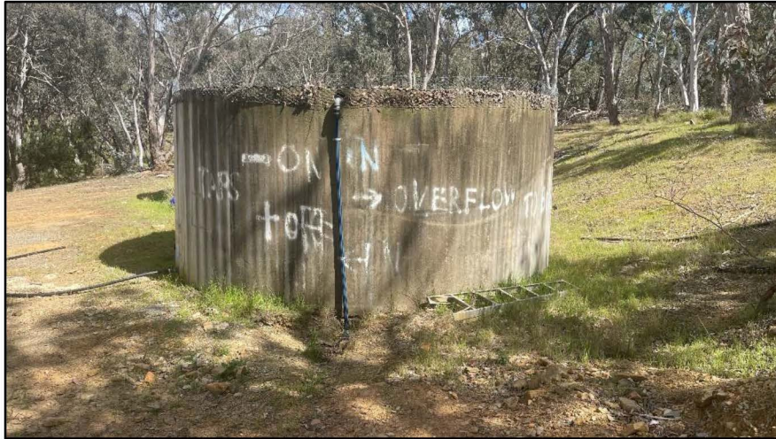
Figure 24a – One of two large concrete water tanks uphill from the underground tank.
