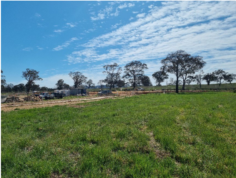
Photo 1: View of Subject Site from near to Blakelys Close Frontage (looking northeast) – Photo credit Adhami Pender Architecture
