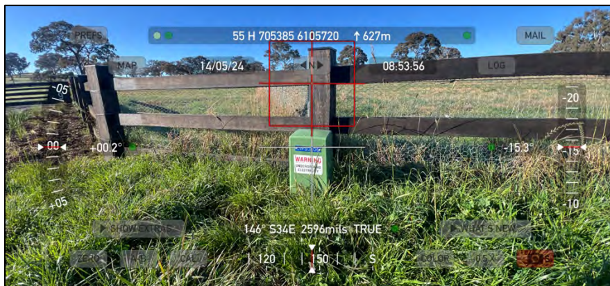
Photo point 6 Looking at underground electricity supplies for the Subject Site.
